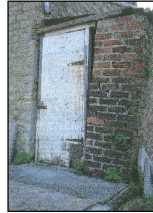
Photograph of lean-to (roof now removed due to collapse)
